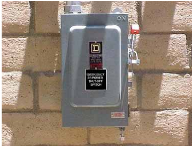
Figure DC 222–5: Emergency RF/Power Shut-Off Switch
