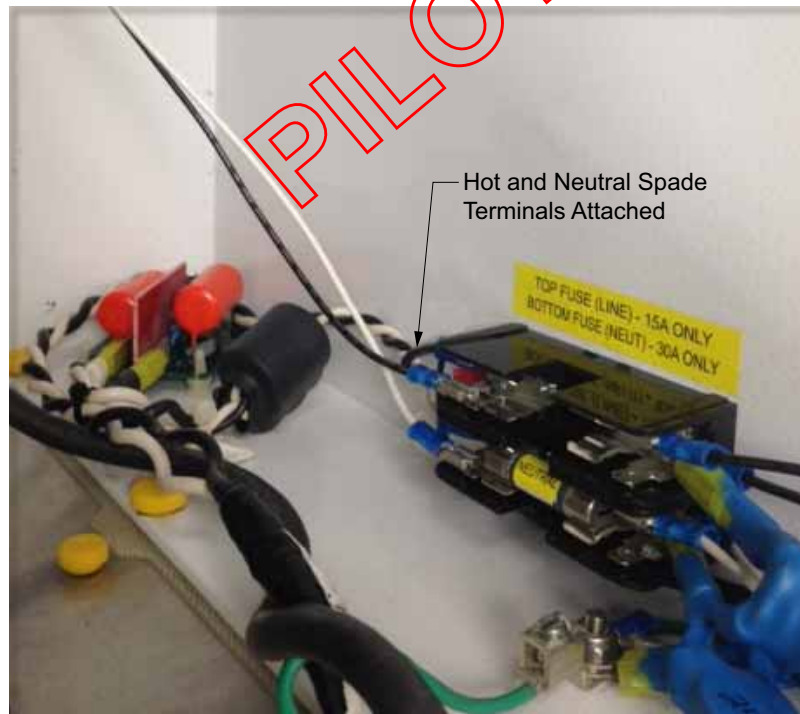
Figure 620P-12: Wiring Harness Cable Terminals Attached
