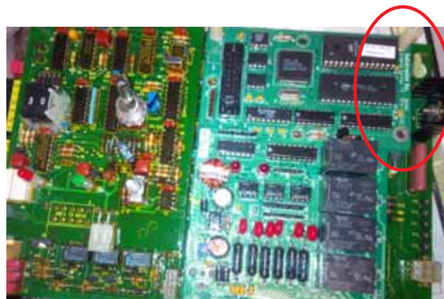
Upon removal of RTU faceplate, RTU Board, right side. Model number detail in-circled in red.
