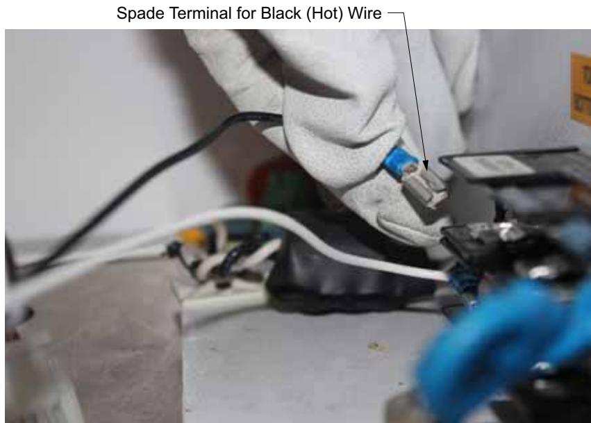
Figure 620P-11: Wiring Harness Cable Terminals Being Attached
