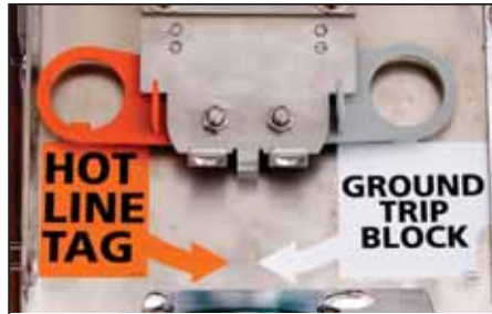
Figure AP 511P-3: Hot Line Tag Lever, Ground Trip Block Lever, and Gang Operated Disconnect Switch Lever
