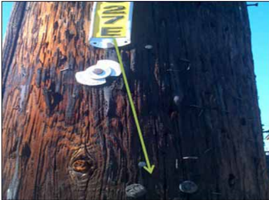
Figure 13.1: Nail Below Pole Tag – Length 50 ft
