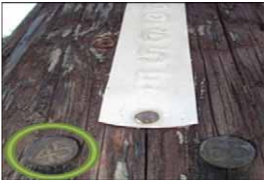
Figure 13.3: Nail Below Pole Tag – Length 45 ft
